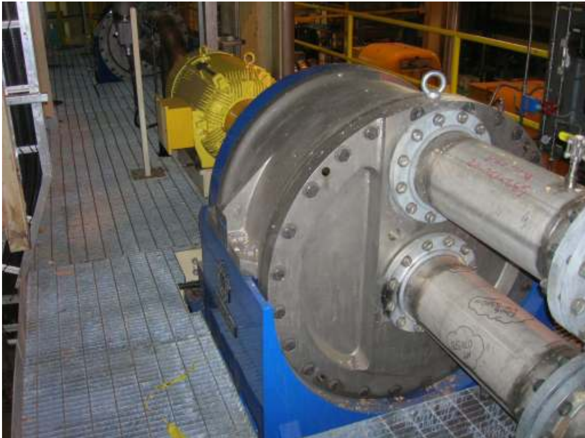
Figure 1. Picture of Fiber Accelerator Installed at ANC
