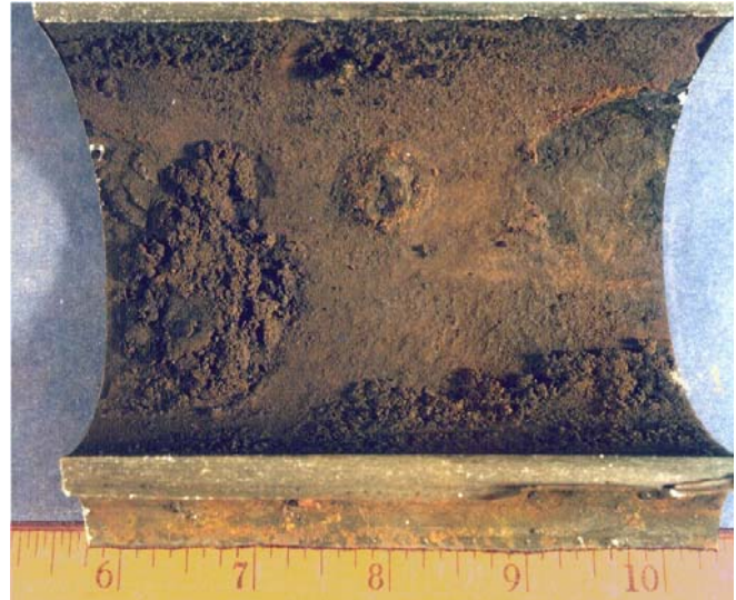
Figure I-3 - Localized Waterside Deposits
