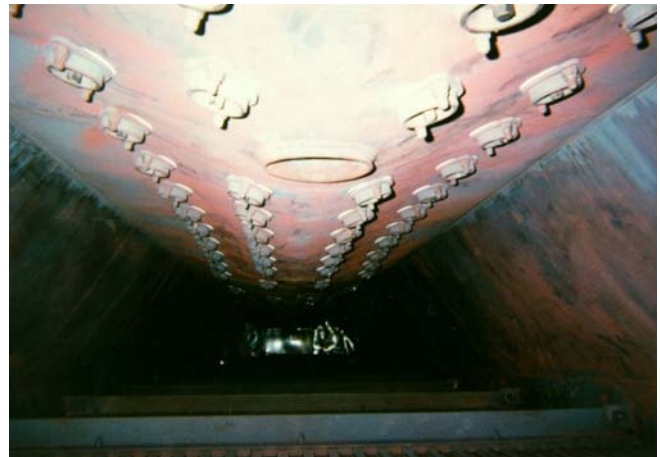
Figure 20 - Deaerator Spray Nozzles And Trays
