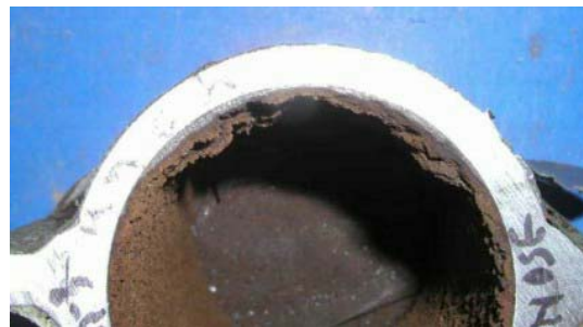
Figure 3 - Boiler Deposit Example
