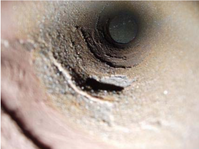
Figure 4 - Boiler Blistering Example
