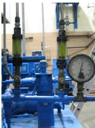
Figure 12. Dryer Bearing Lubrication System.
