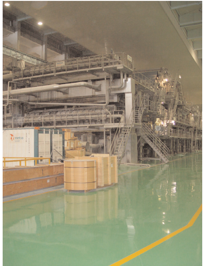
Wet end of the new PMI containerboard machine.
