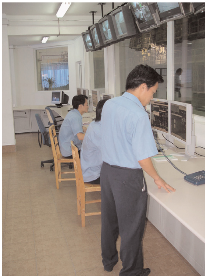
Workers in the control room for PM1.
