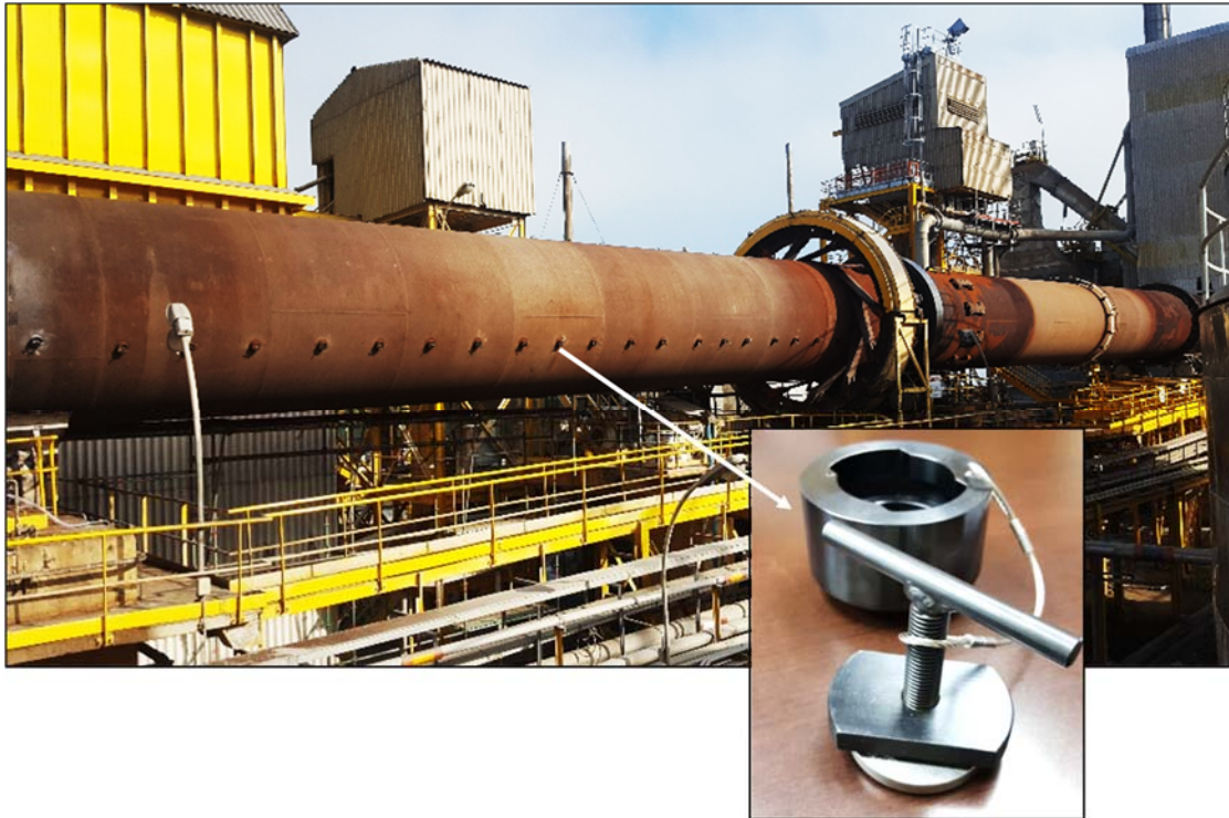
Figure 3. Sockets over the shell in the lime kiln.
