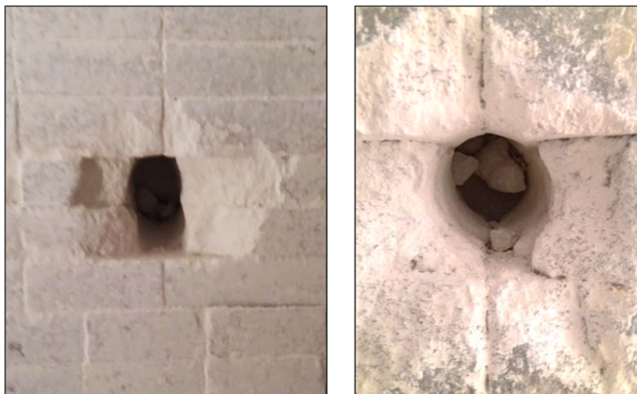
Figure 10. Brick damage incurred during drilling.
