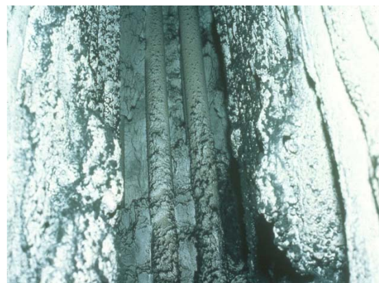
Figure 18. Complete plugging at the generating bank inlet
