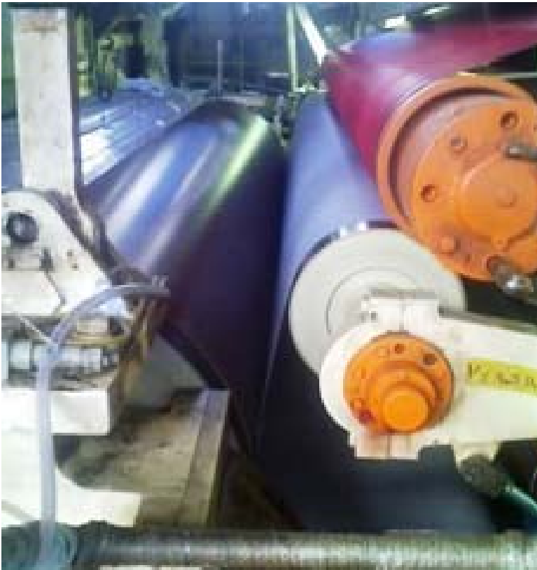
Hose to collect vapors from above the paper web
