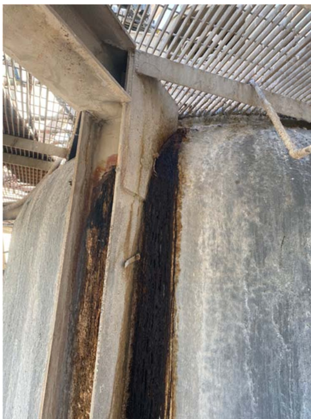
Figure 2 Cooking liquor leak originates behind the digester structure support beam.
