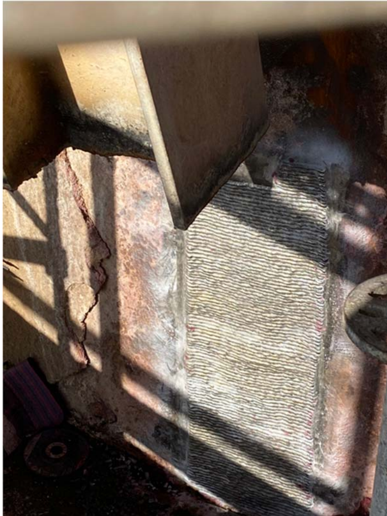
Figure 3 ASME Code repair of exterior CUI found behind a structure support beam.
