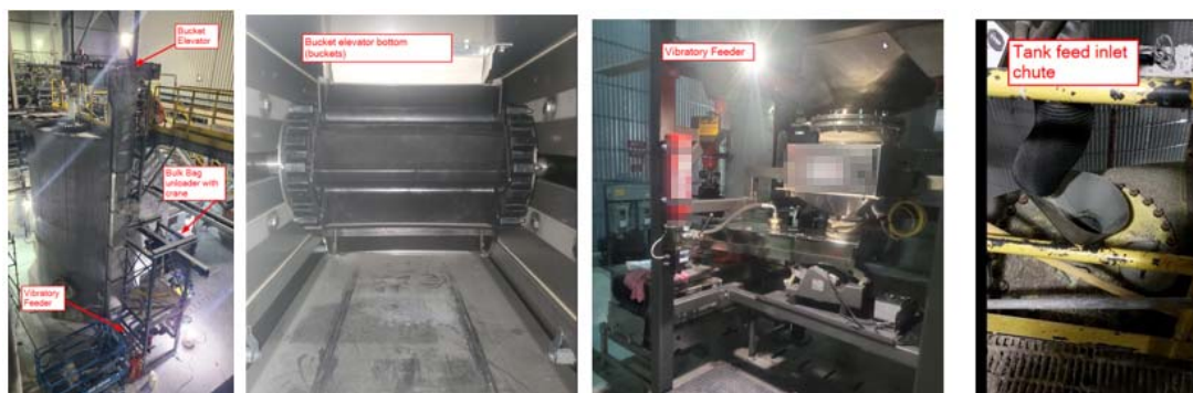
Figure 13 Sulphur addition system
