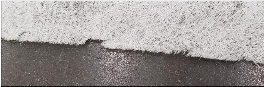
Fig. 4 Example of torn edges.
